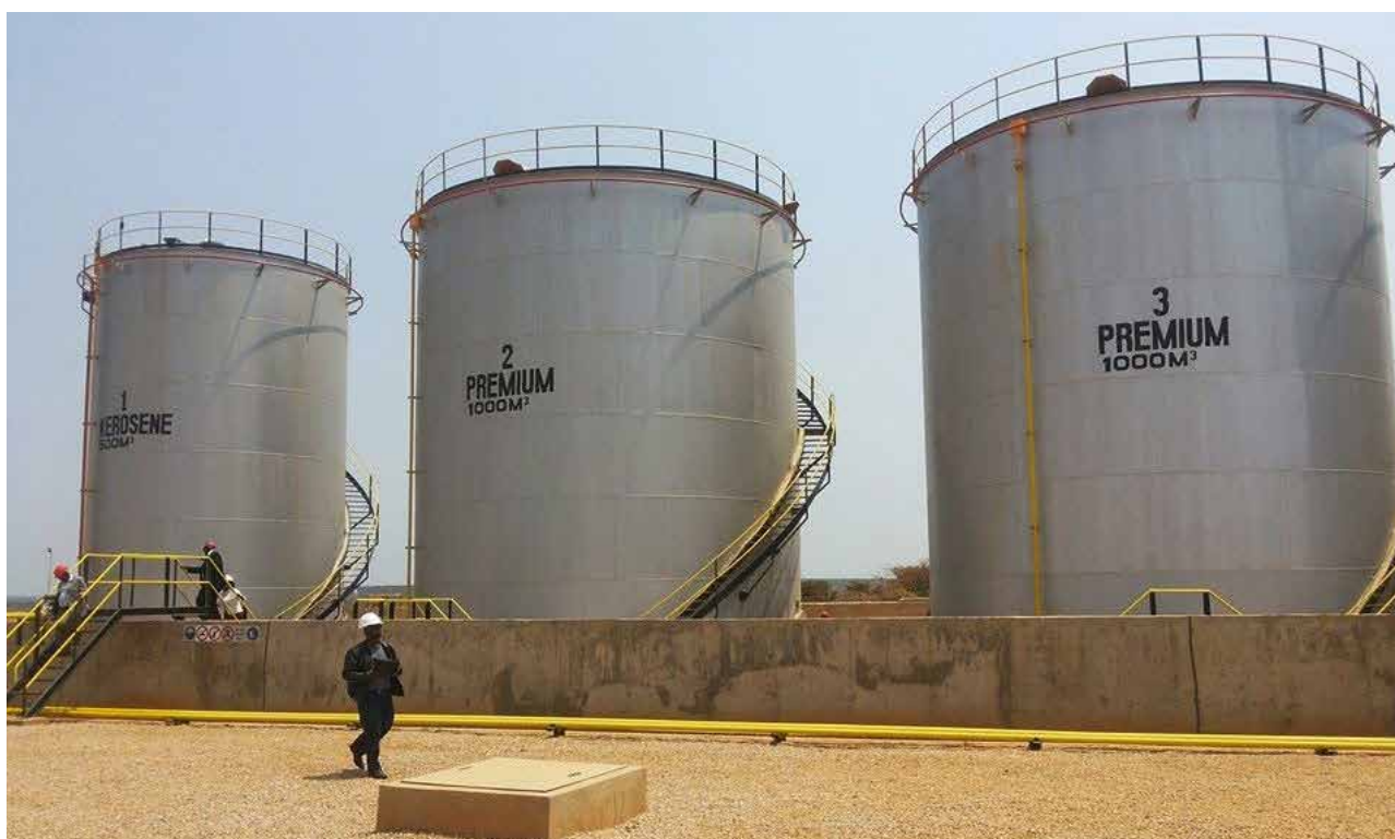
Mpika Fuel Depot Source: TAZAMA Pipelines Limited
